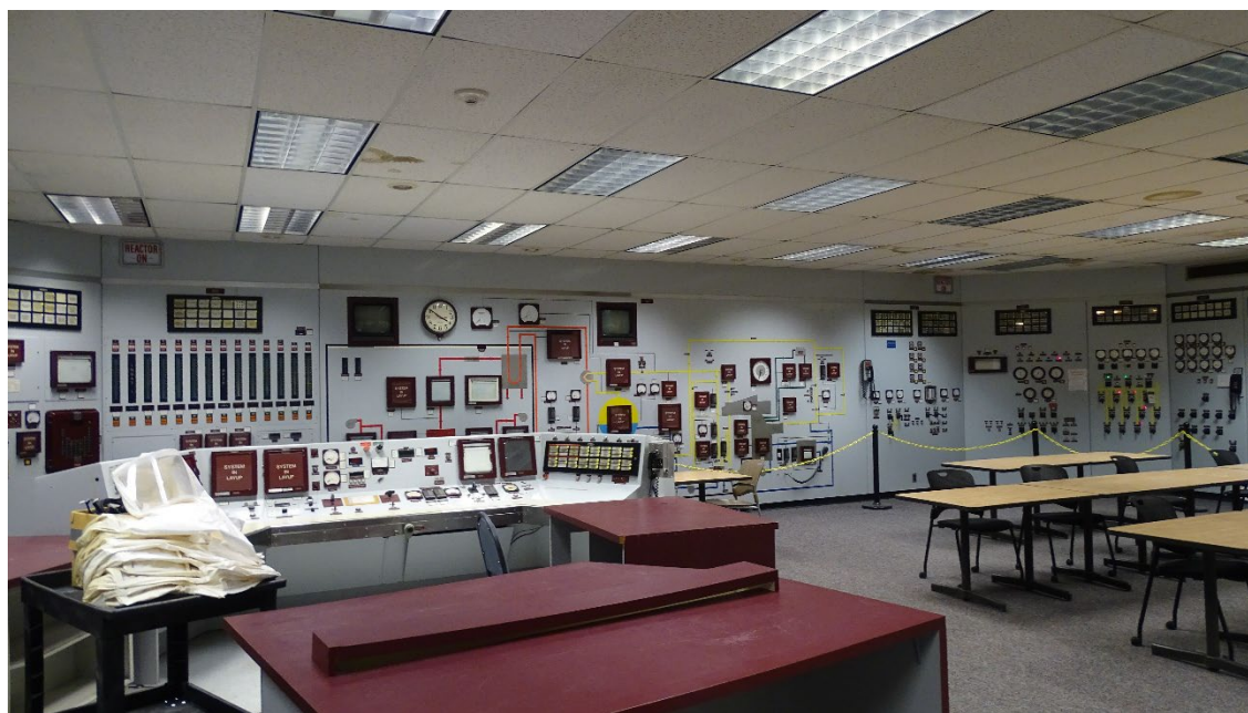
Figure 8. Overview of control room (INL CRMO 2024).
