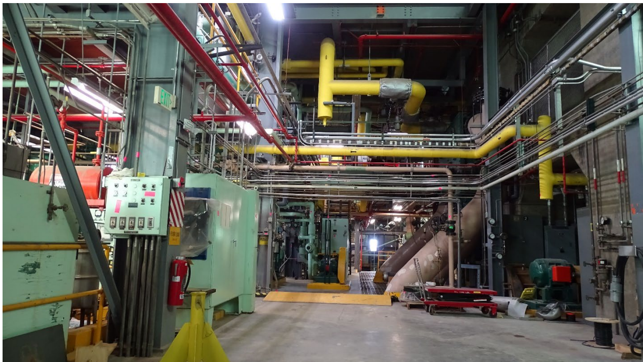
Figure 5. Interior of MFC-768 showing piping for steam system (INL CRMO 2024).
