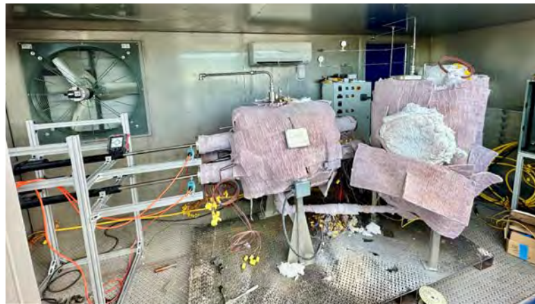
HITB thermal energy storage facility with insulation in a cargo shipping container located at INL Engineering Demonstration Facility.
