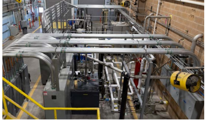
Support facilities for the HTE capabilities (electric distribution systems, boilers, water desalination system, etc.) at the HTTF.
