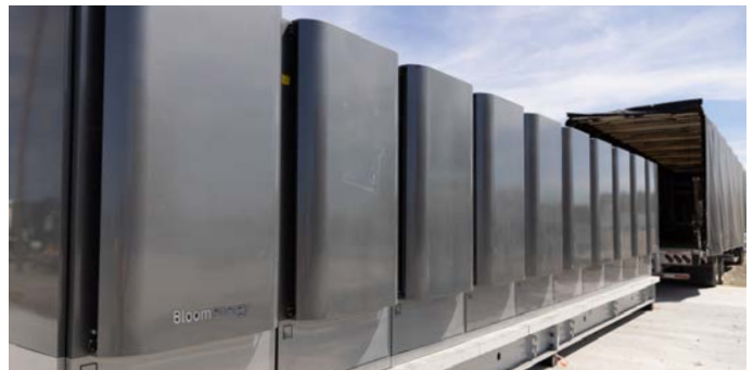
Installation of an HTE system at the HTTF.
