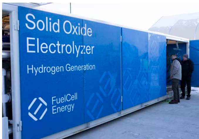
FuelCell Energy's 250 kW HTE system being tested at INL's Energy Systems Laboratory.
