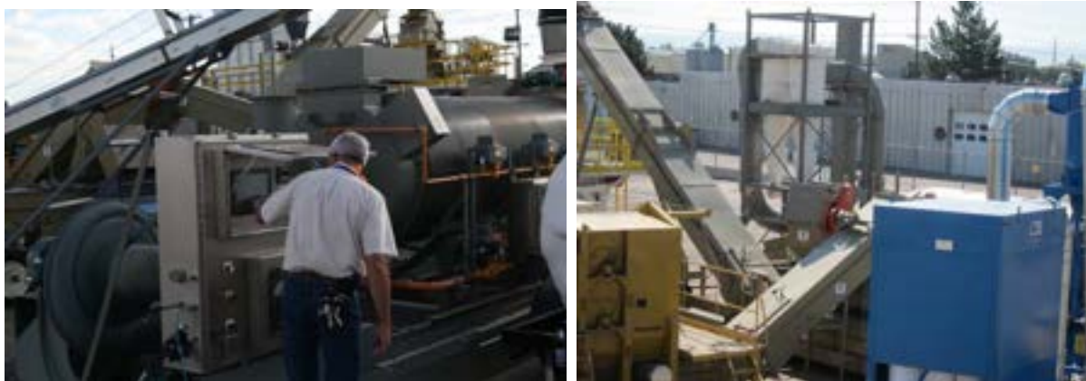
Figure 5. The control screen near the dryer burner (left). Dried wood material is returned to the conveyor that moves the ground herbaceous materials (right).
