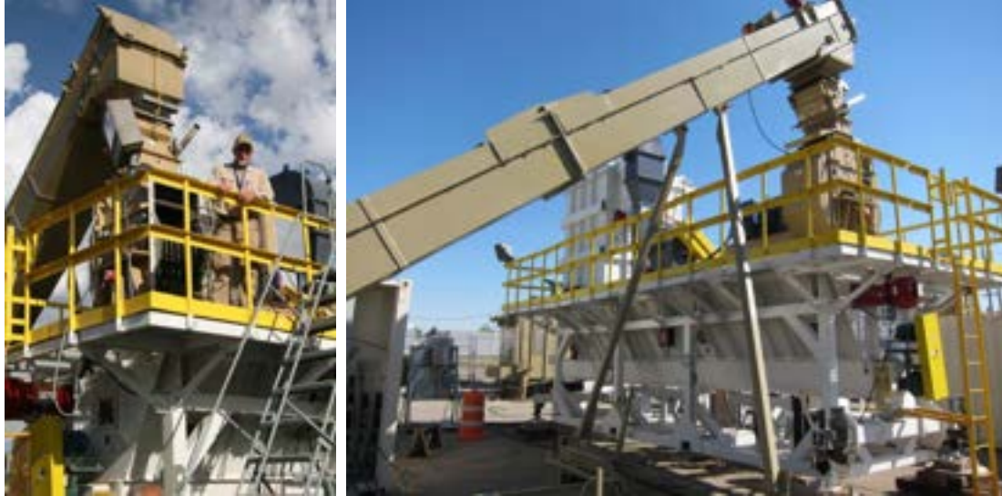
Figure 6. Hammer mill mounted on top of the plenum chamber (left). View showing the inlet conveyor, hammermill, blower (dark gray), and bag house (white) mounted on a platform above the plenum chamber (right).
