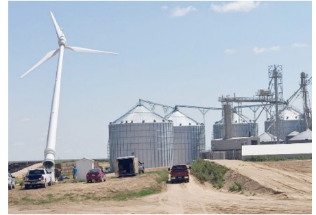
A 25 kW wind turbine serving Champion Valley Feedyard, a cattle operation in Yuma, CO, undergoes maintenance [1].
