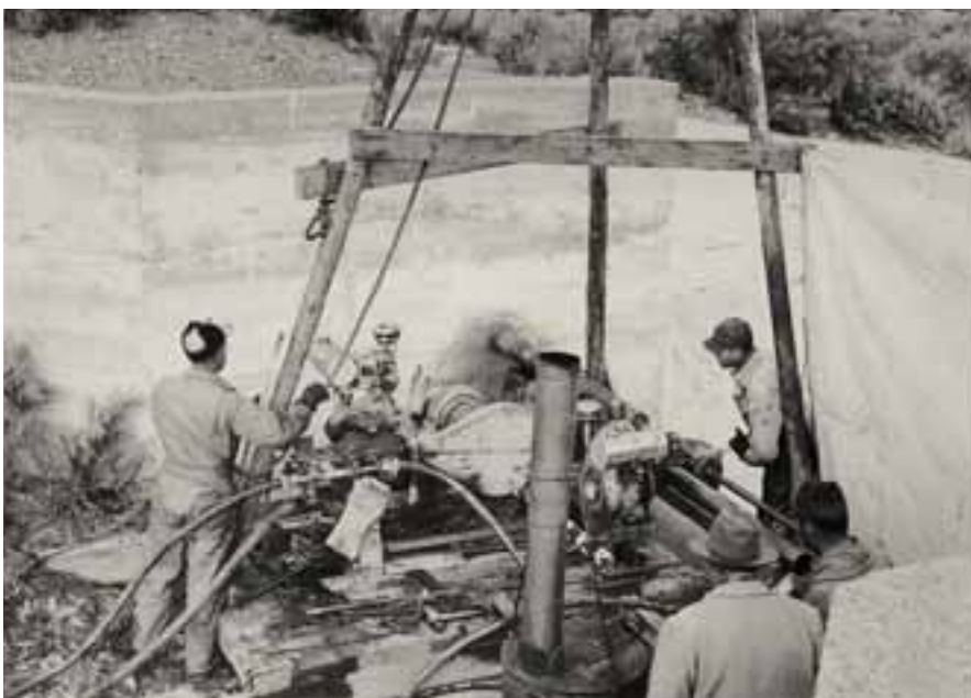
Drill rig crew takes core sample from spillway on an old irrigation canal.
