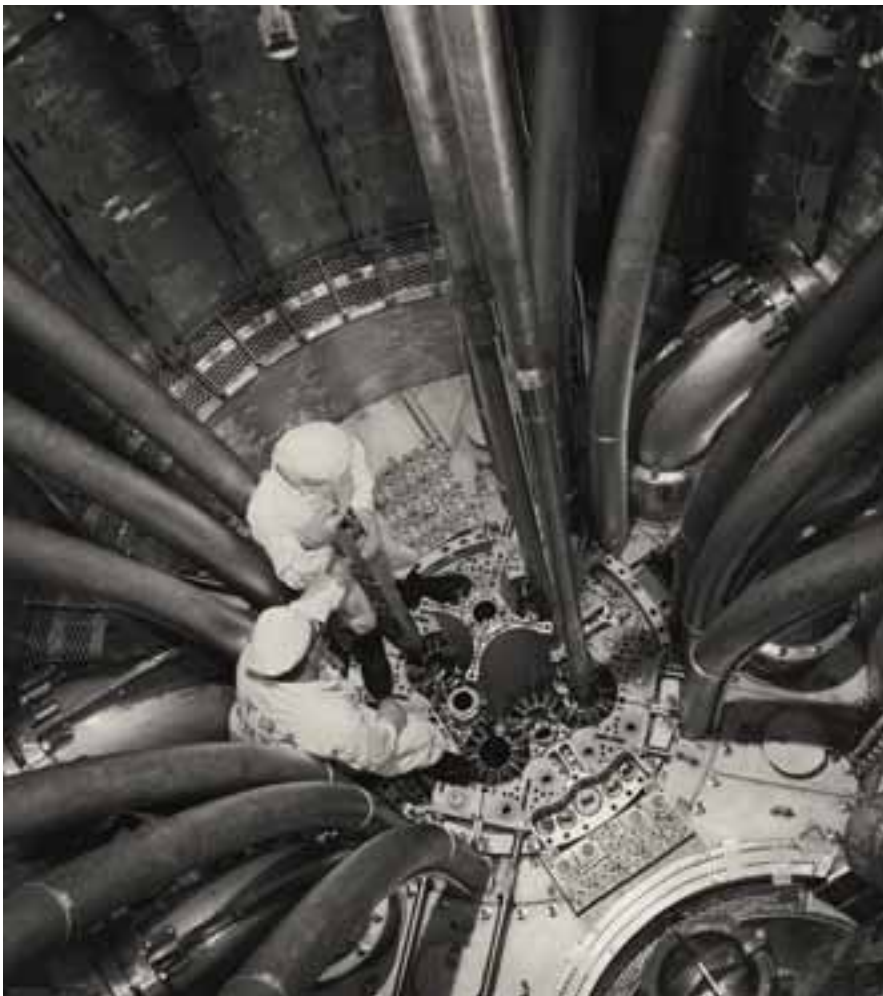
ATR technicians check the fit of a dummy fuel element in the reactor core (before ATR became operational). The curved pipes are for instrument leads and reactor coolant. The vertical pipes provide paths for experiments into the core area.
