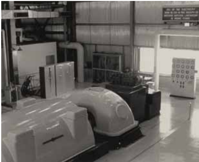
EBR-II turbine generator.
