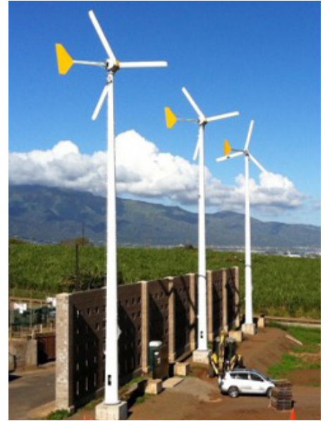
Central Maui Landfill Refuse and Recycling Center 10 kW wind turbines in Hawaii, installed in 2015. Source: Cliff Ryden.
