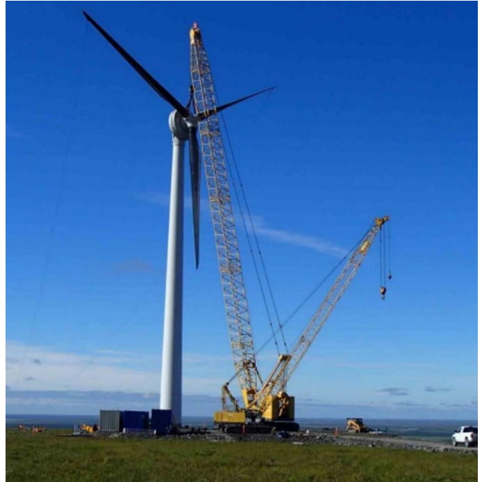
The 900 kW wind turbine constructed in Pitka's Point, AK, serving three local communities, helps offset diesel fuel use and mitigate risk of fuel shortage [1].
