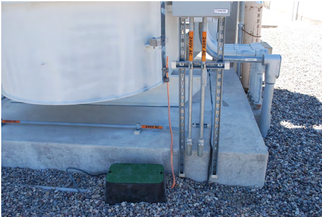
Figure 2. Typical INL transformer—GMD ground current measurement.
