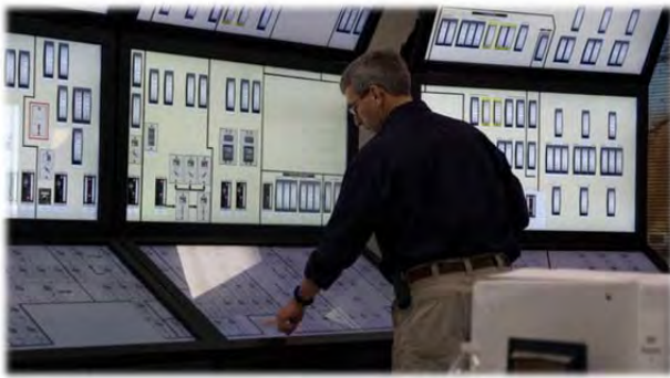
FIGURE 1. Touch screen benchboard panels.
