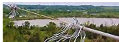
Figure A-75. Damaged conductor following the 2013 tornado.
