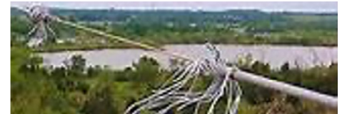
Figure A-75. Damaged conductor following the 2013 tornado.
