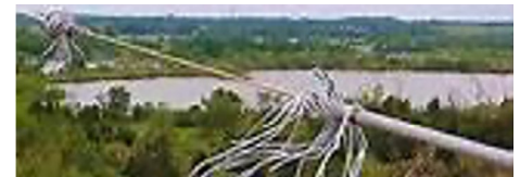
Figure A-75. Damaged conductor following the 2013 tornado.
