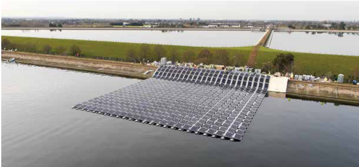
Source: © Lightsource BP Floating Solar Array, London.
