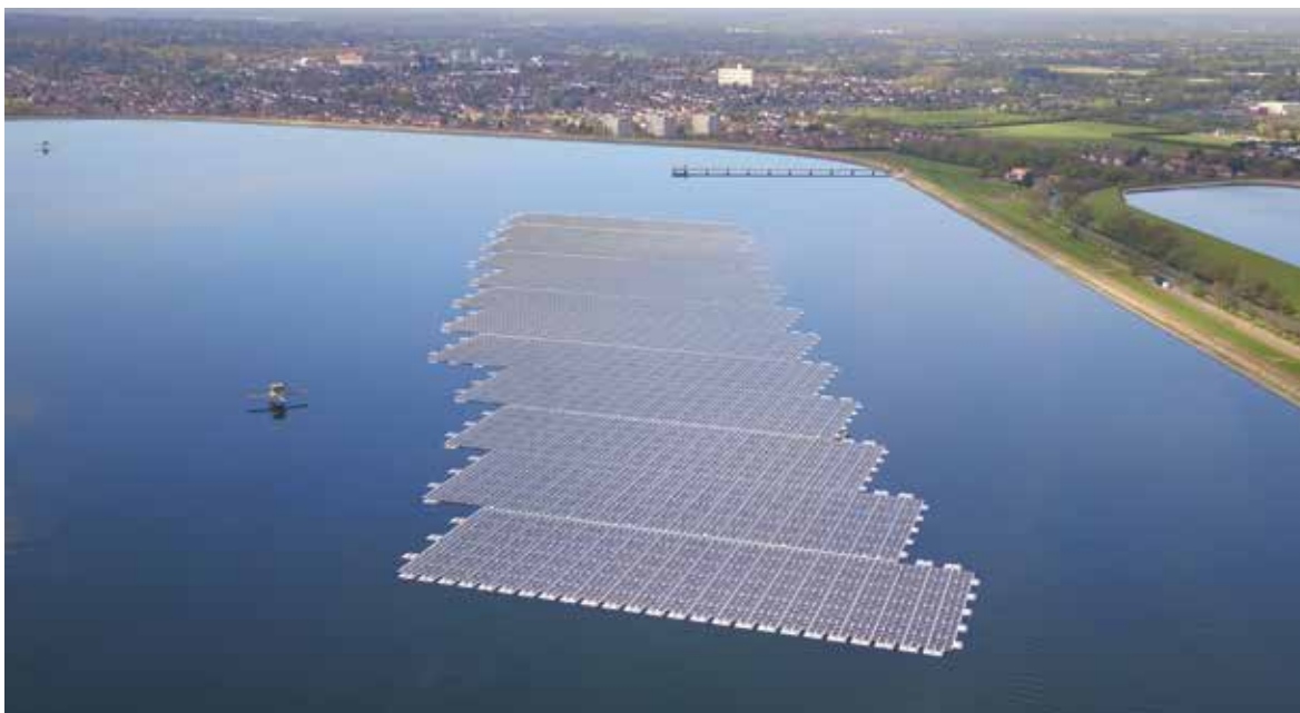
FIGURE 3.13. FPV project on the Queen Elizabeth II Reservoir, United Kingdom
