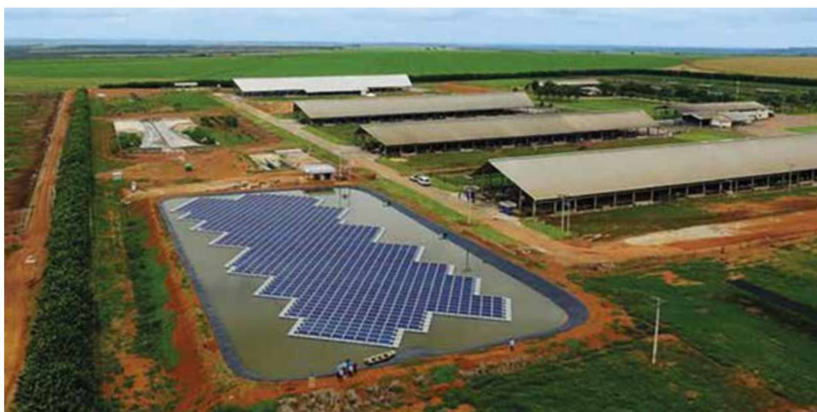
FIGURE 3.4. FPV system (of 305 kWp capacity) in Goias, Brazil
