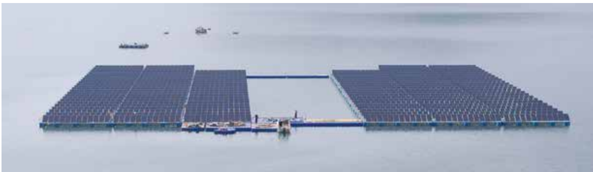
FIGURE 6.5. LSIS FPV installations in Korea
