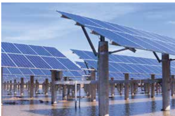
FIGURE 1.5. A “PV over water” installation
