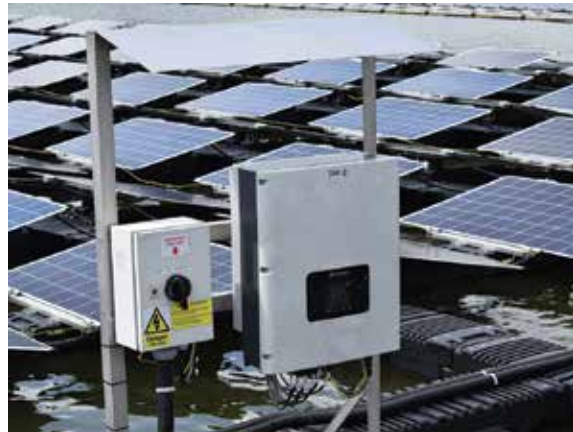
FIGURE 2.14. String inverters placed on the floats together with PV arrays
