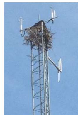
Figure 4-2. Raven nest on one of the two NOAA towers.
