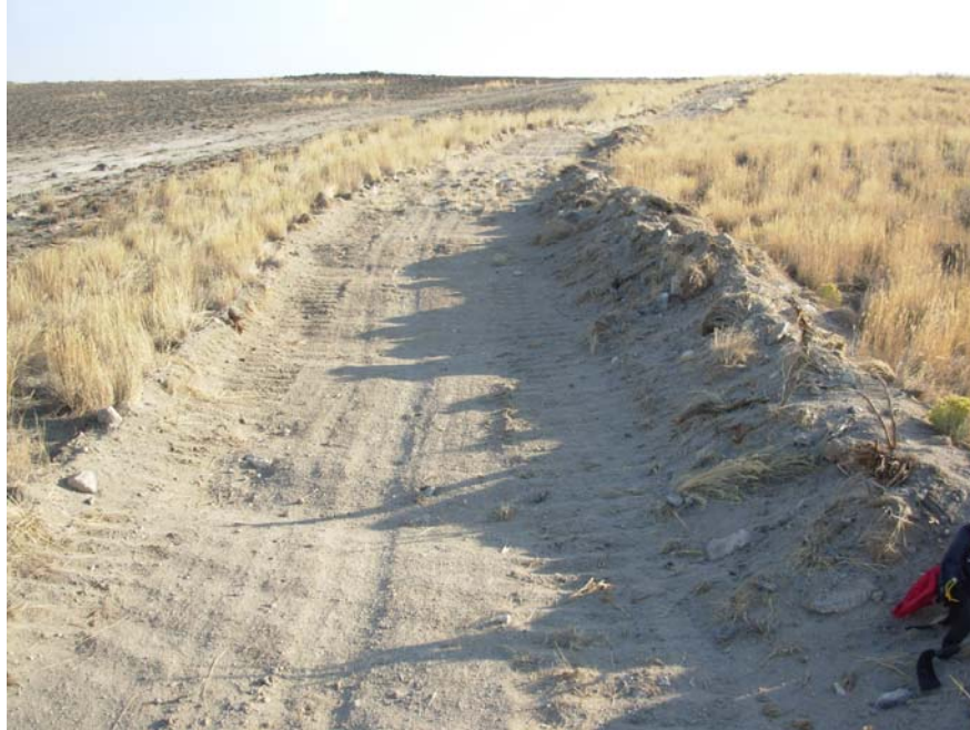
Figure 4. Containment line on Highway 20 Fire with large rick and bladed deep enough to remove all vegetation.
