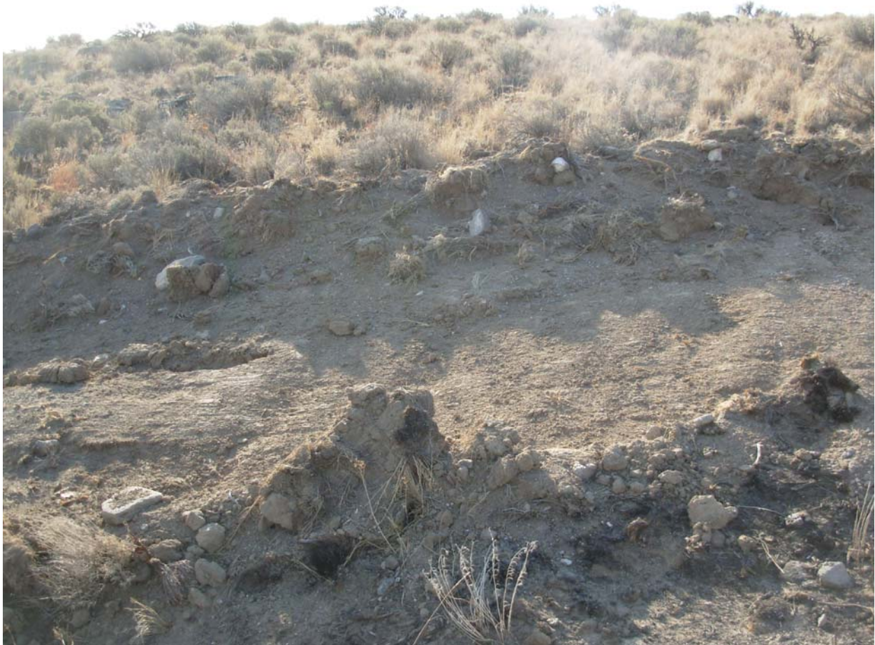
Close-up of damage on steep side hill. These ricks should be pulled in on both sides and re-contoured to match surrounding terrain.
