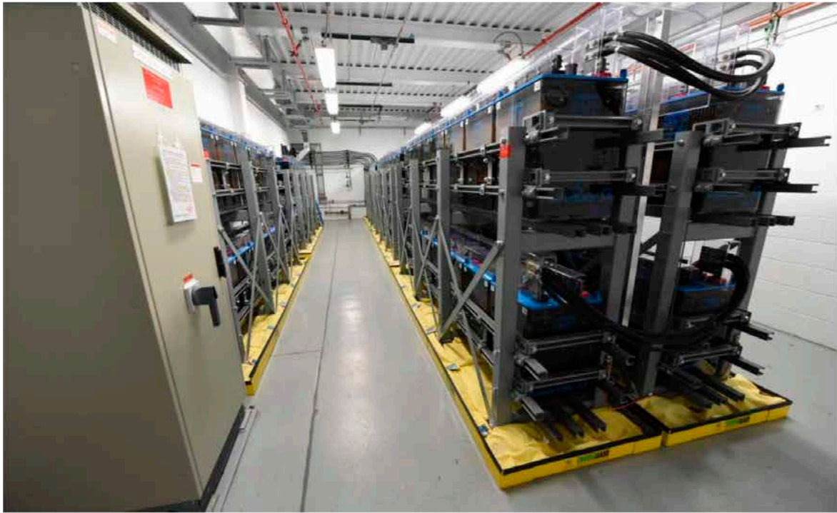
Figure 3-1. Commercial Utility Power with Uninterruptible Power Supply at the ATR Complex.
