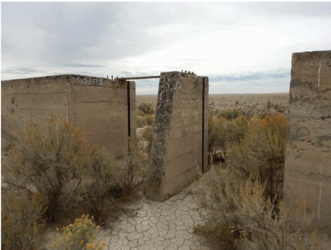
Figure B-2. Lateral 6 Looking Southeast to Gate Structure with Main Owsley Canal Running East-west on the Second Owsley Project.
