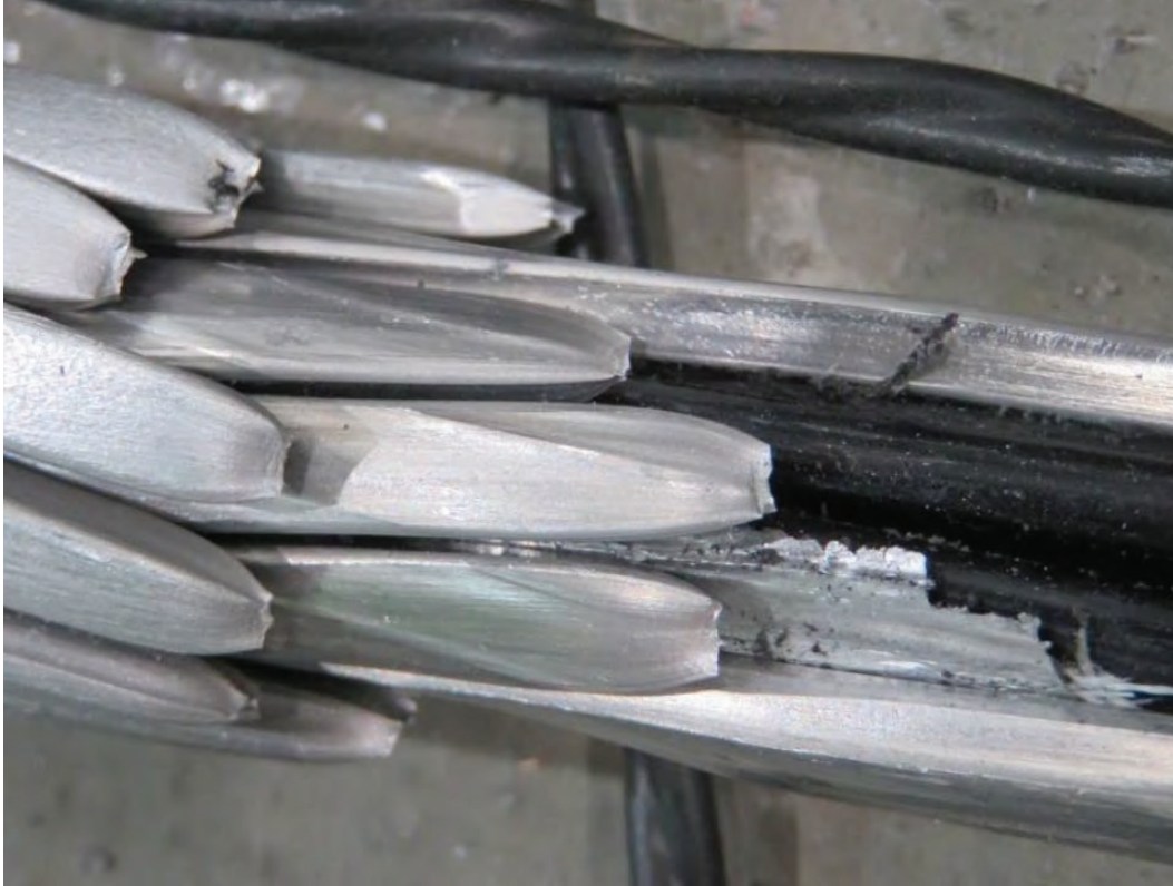
Figure 3-14. Appearance of Celanese ACCS C 7 -TW aluminum strands after failure
