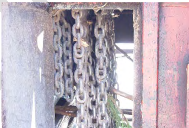
Figure 2-54. Flail shredder screen in Greenville, Alabama. The screen stops larger pieces from passing through the flail (Photo credit: Christopher Wright, INL, July 2010).
