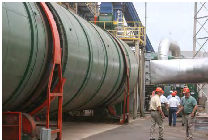
Figure 2-74. Rotary drum dryer used at a wood processing facility (Photo credit: D. Brad Blackwelder, INL).
