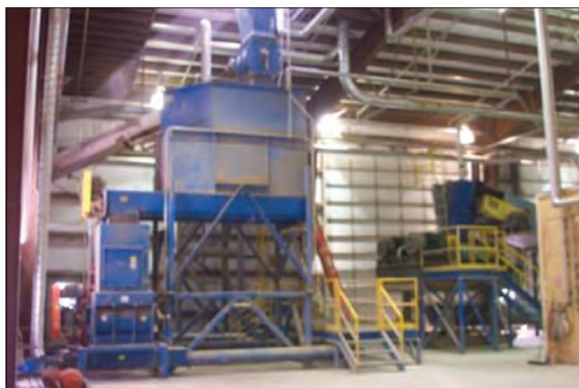
Figure 2-33. Biomass feed system for a biochem or low-pressure thermochem conversion processes, including the evenflow metering bin (large blue elevated bin) and the augers and pneumatic conveyance equipment that enters and exits the metering bin (Antares, 2008).
