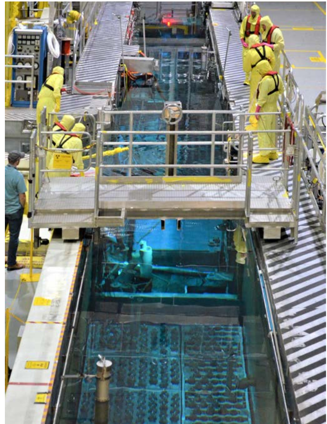
Figure 9. ATR storage canal.
