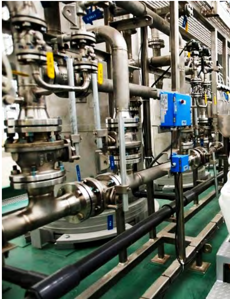
Nuclear power plant field sample
