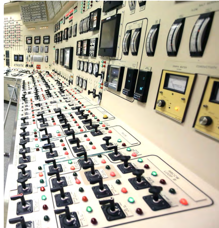
Nuclear power plant main control room
