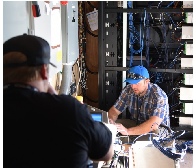
C3D gives utilities time to defend against a cyberattack by limiting protective relays' exposure to outside communications while maintaining operations.
