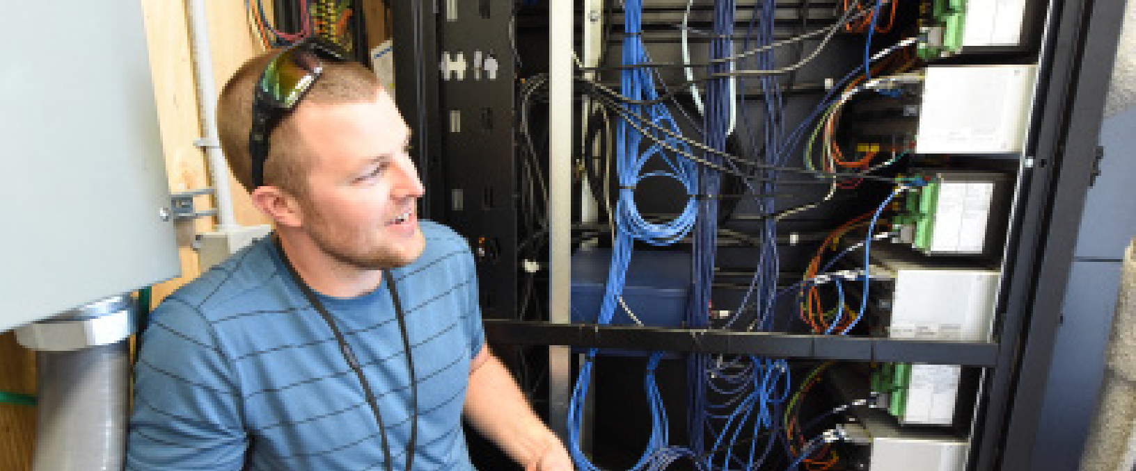
INL engineer Dylan Reen installs a Constrained Communication Cyber Device to a protective relay.
