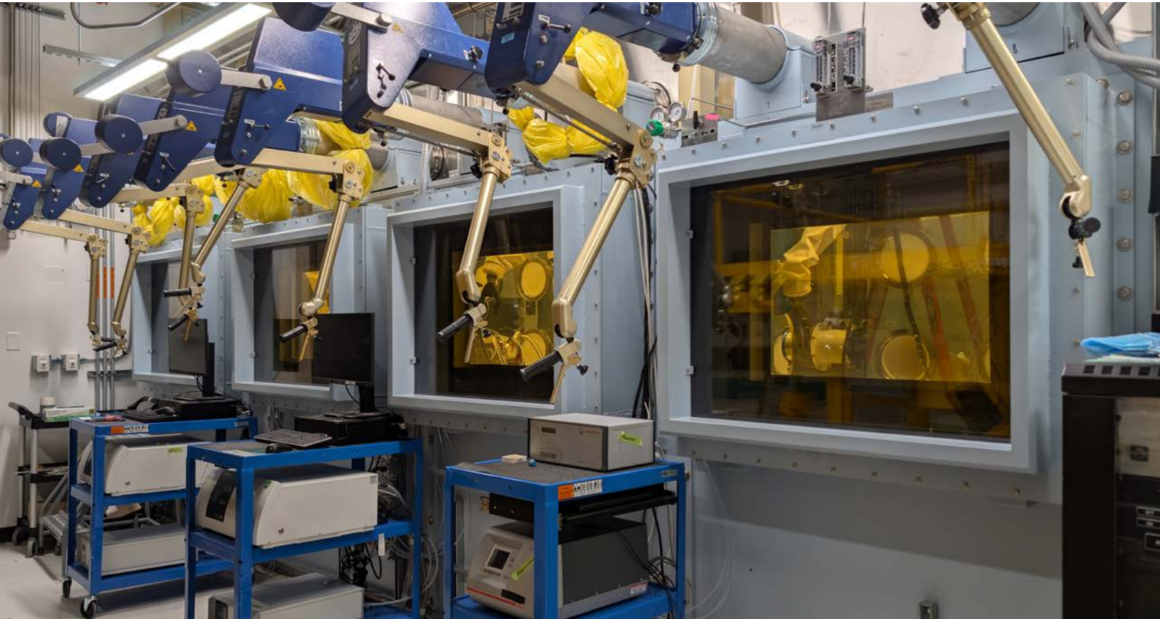
MSTEC shield hot cell with manipulators and characterization equipment controls for working with irradiated samples.
